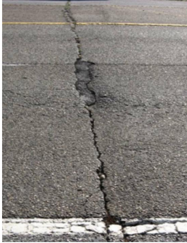
Figure 3: Sample Transverse cracking (Dong, 2013)
