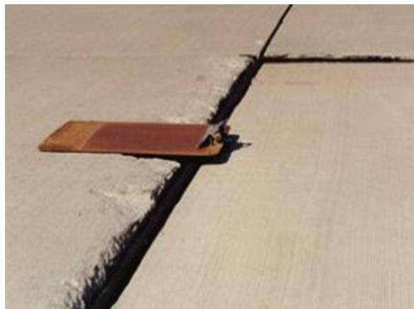
Figure 5: Sample of faulting (Iowa Airport Pavement Management System, 2020)
