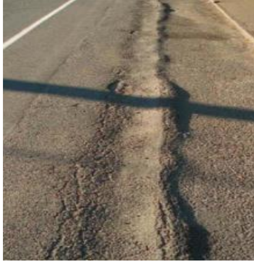
Figure 4: Sample of the rutting (Fussl, 2014)
