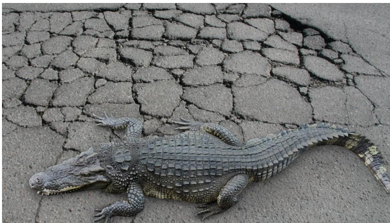
Figure 1: Sample of alligator cracking (J.Mrugacz, 2016)
