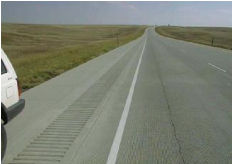
Figure 2: Sample of Longitudinal Cracking (Ardani, 2003)
